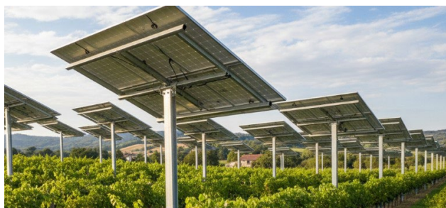
Figure 2. Stationary method of mounting a solar panel on a support above the ground.
